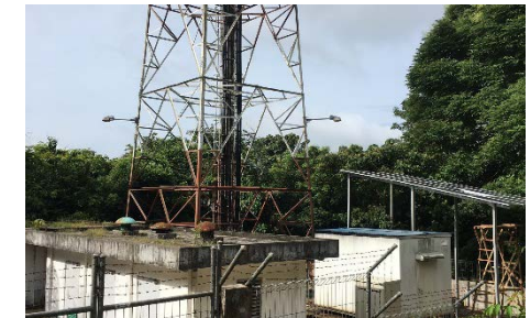
【Low carbonization of mobile communication station】 (Indonesia) 146t Start operation: Apr. 2017
