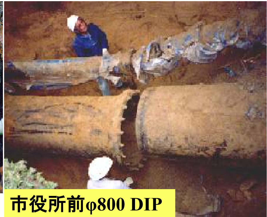
Ductile iron pipes (DIP)
