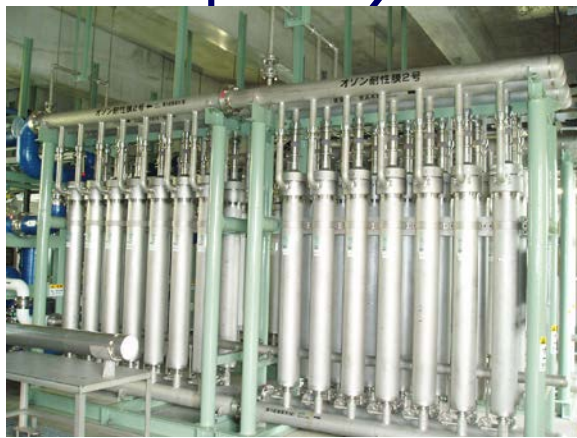
Shibaura Sewage Treatment Plant Membrane technology
