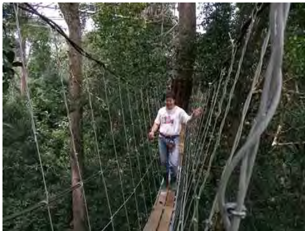
Canopy walkway for the observation of arboreal animals and plants (under construction in pasoh Forest in the State of Negeri Sembilan, Malaysia).
