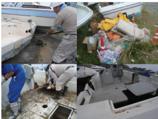
Fig. 7 Decontamination (removal and washout of materials or sediments) of boat wastes in Soma, Fukushima.
