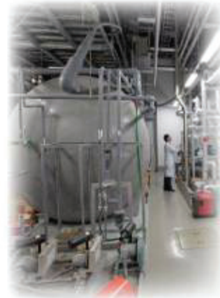
Johkasou system for domestic wastewater treatment
