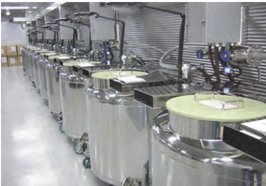
Liquid N 2 vapor-phase storage tanks installed in the Environmental Specimen Time Capsule Building
