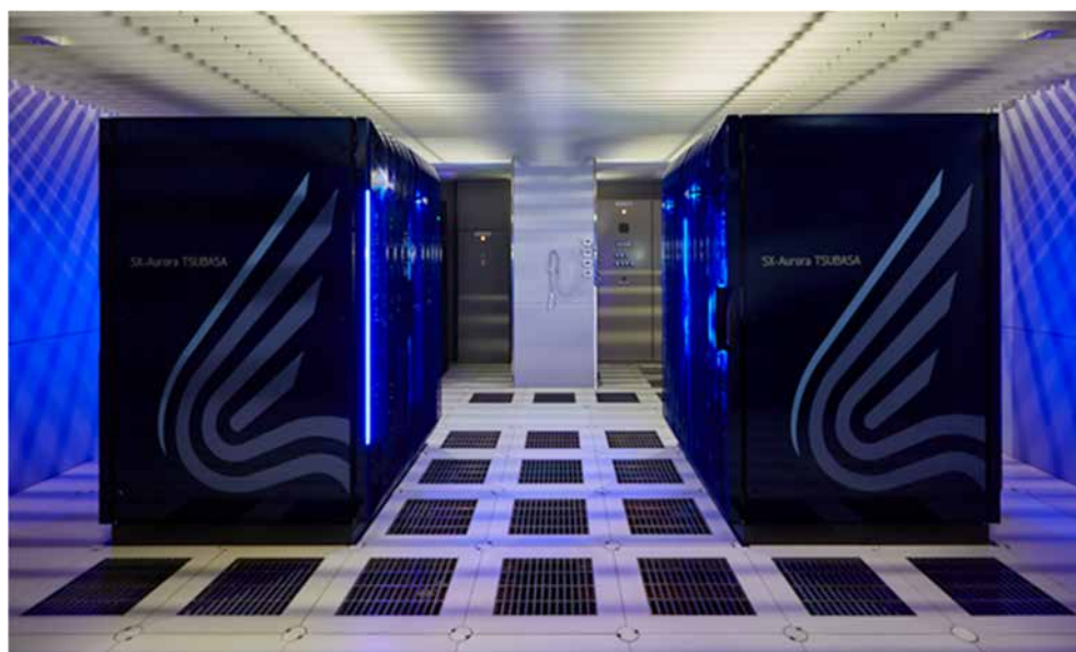
Fig. 1 The NEC SX-Aurora TSUBASA supercomputer
