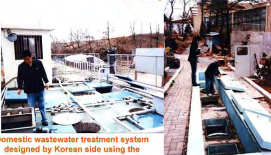
Small scale restaurant wastewater treatment system designed by Korean side using the project's results
